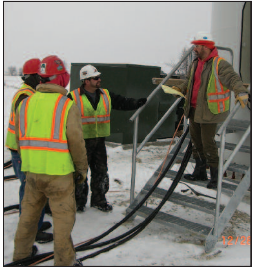
Employees hold their daily on-site safety meeting at the base of a wind turbine.
